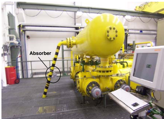
Figure 10: Photograph of the installed three-dimensional vibration absorber.
