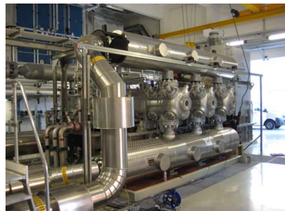
Figure 13: 1 st stage of the 6-cylinder reciprocating compressor plant with VFD-driven e-motor drive.
